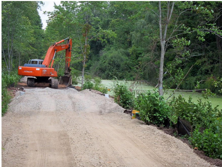
Construction of the trail in Cheshire Connecticut, between West Main and Jarvis Streets, fall 2015
